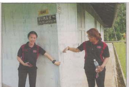
Jong (left) and society secretary Pauline Menggong show the old bellan post which has served as a structural support for a building at the settlement since 1925.
