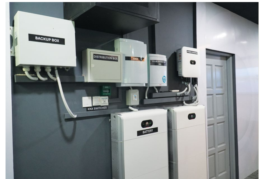
Figure 4: Physical Setup of the PV Solar System Components.
